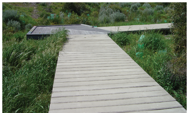
A pre-cast concrete boardwalk can be integrated with timber elements, such as here at Secret Harbour in south-west WA.
