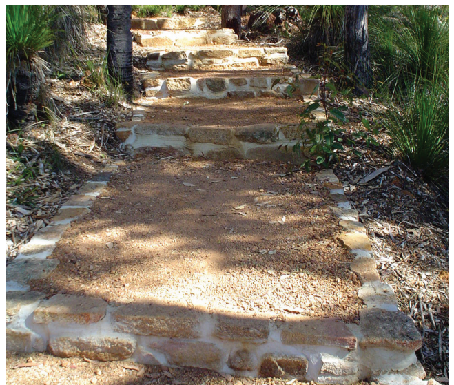
Quality construction, such as these rock steps on the Golden View Trail in Kalamunda (WA), is the hallmark of a quality trail.
